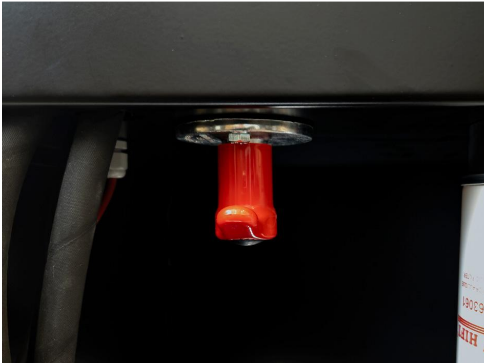
Figure 3. Switch in the ON position
